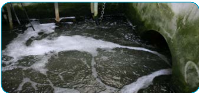
In the outlet: VisoTurb® 700 IQ F turbidity sensor with ultrasonic cleaning
